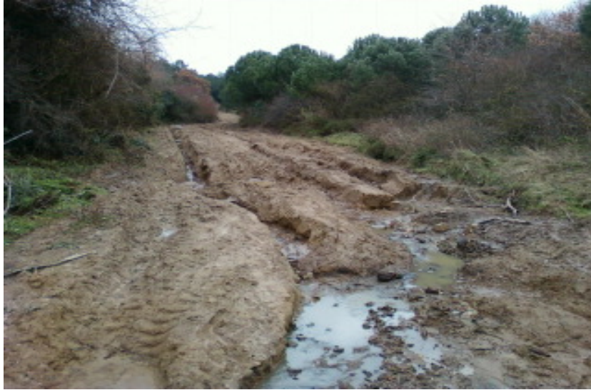
Figure 26. Poor condition earth road.
