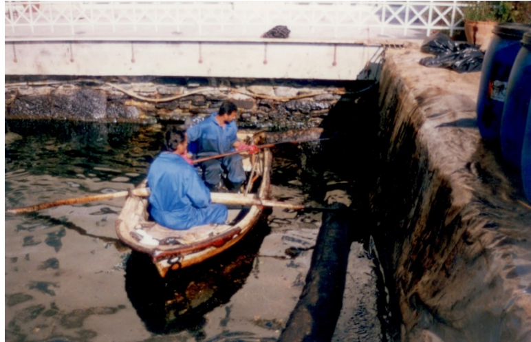
Photo 2. The oil slick contaminated the infrastructures including piers, seawalls and waste barriers (photo by S.Ünlü).
